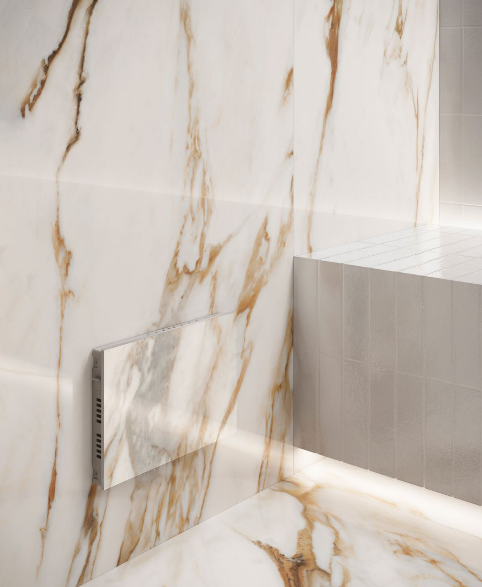
Inside Camouflage / steam generator /
